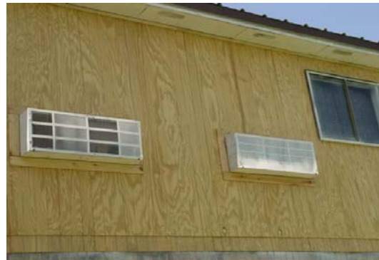
Lender Required Repairs / RUSH
